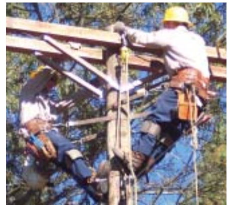
At the Open House, City electric line workers will demonstrate pole top rescue and team pole climbing skills that have gained them statewide recognition.
