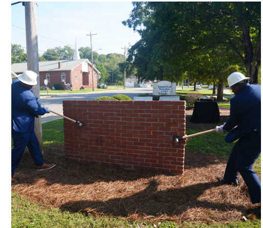
Councilmembers Derrick L. Lindsay and Perry L. Sutton commence the renovation of the McGirt Auditorium in September 2023.
